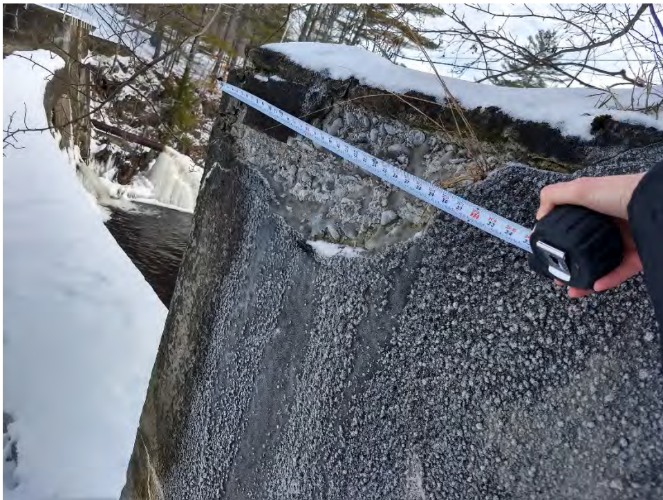
Photo No. 10 – Upper Dam – Upstream side of right abutment retaining wall. Note spalling concrete.
