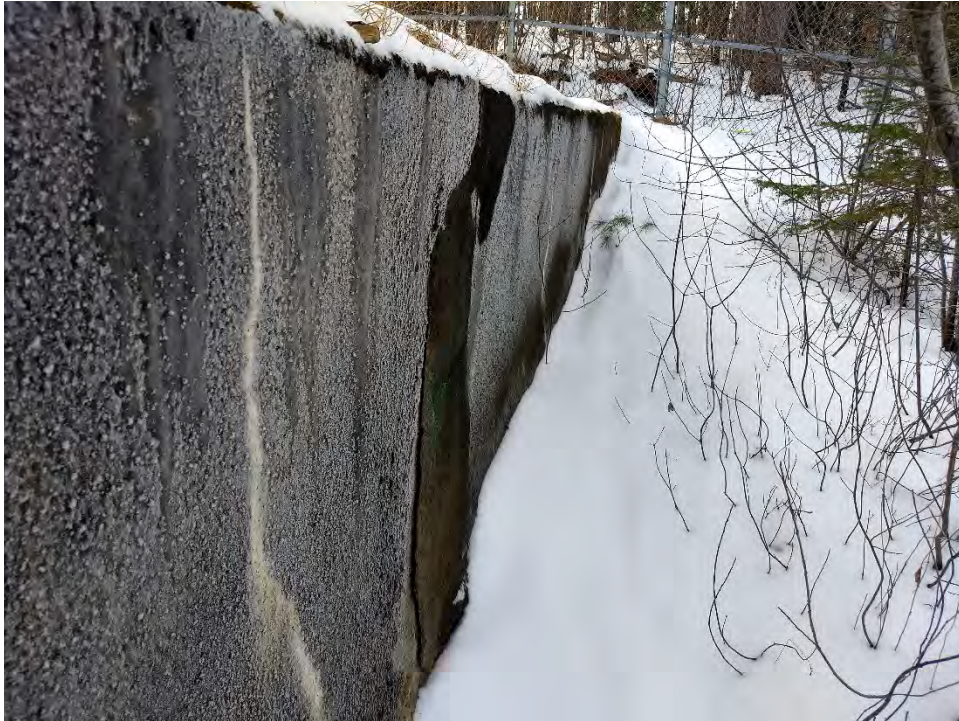
Photo No. 11 – Upper Dam – Right abutment retaining wall, looking right. Note cracking and failing concrete repairs.
