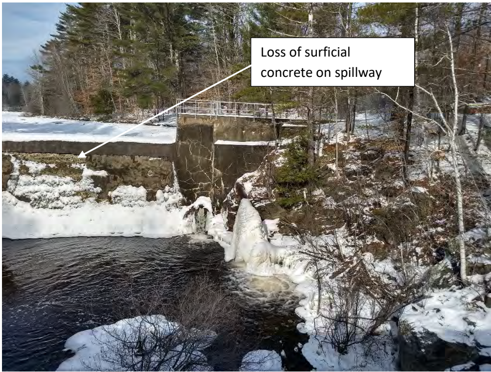
Photo No. 4 – Upper Dam – Downstream side of left abutment and spillway. Note cracks in abutment and loss of surficial concrete on spillway.
