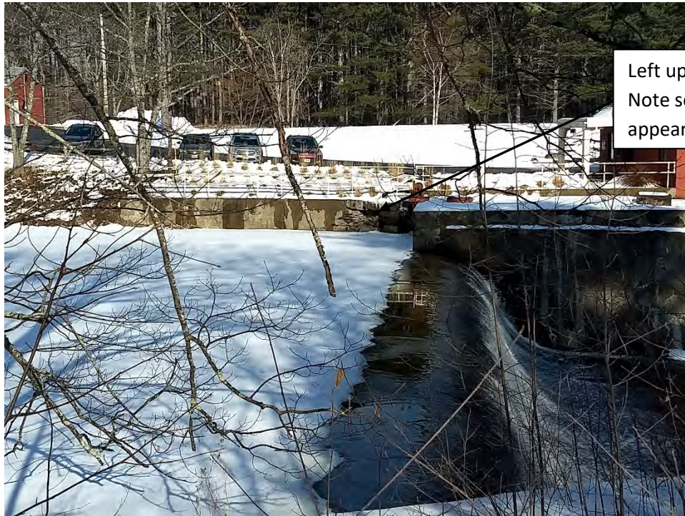
Photo No. 23 – Lower Dam – Upstream left abutment training wall. Note section where concrete facing appears to have failed.
