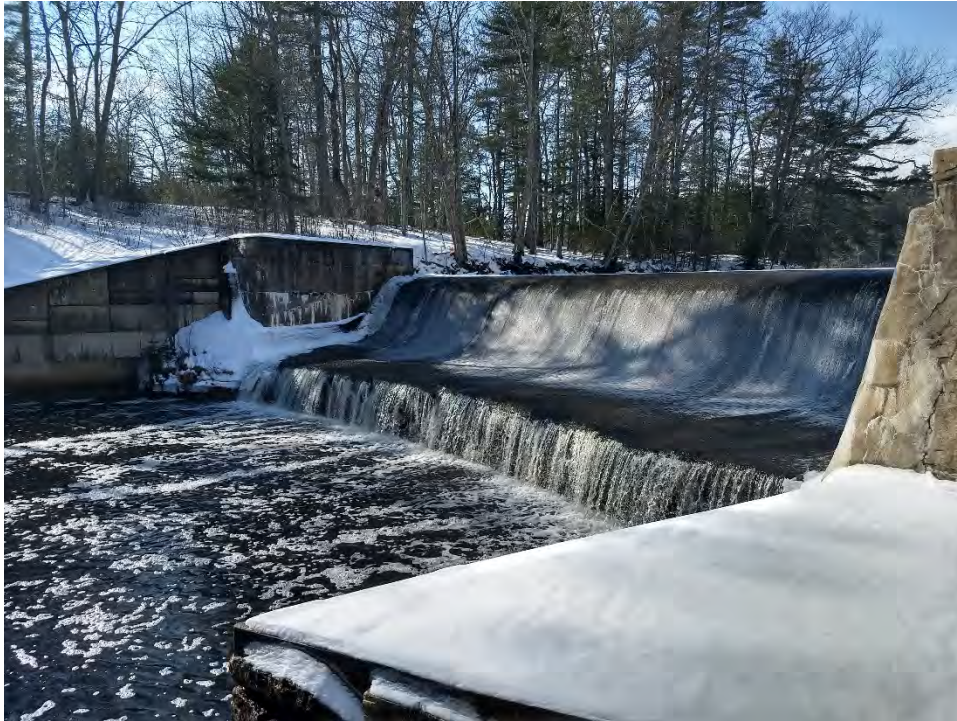
Photo No. 15 – Lower Dam – Downstream side of spillway. Note spilling by a couple of inches, vegetation on right downstream toe.
