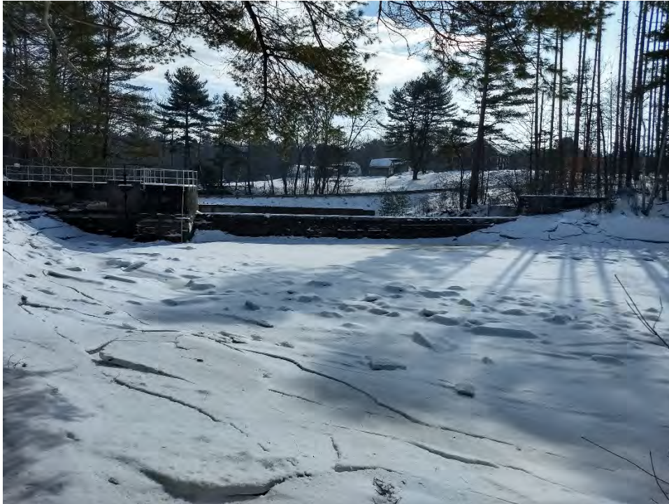
Photo No. 5 – Upper Dam – Upstream face. Note reservoir approximately 6' below spillway sill.
