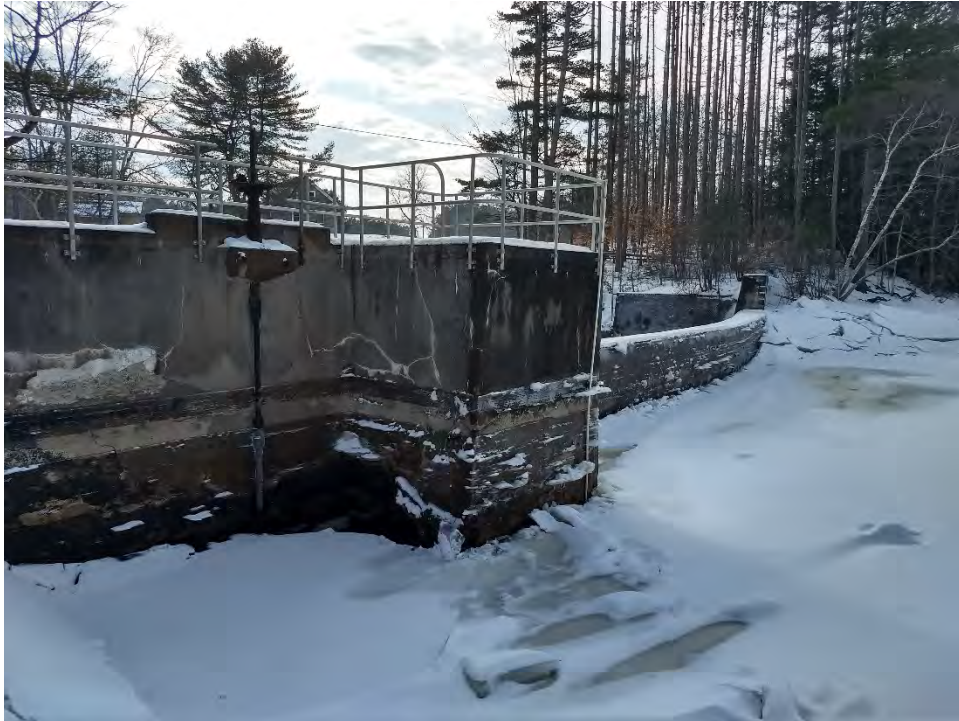
Photo No. 7 – Upper Dam – Upstream side of left abutment and spillway. Note ice against spillway face.
